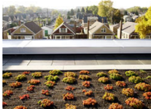
Top Soil On the third-story roof of Tarkington Elementary School, in Chicago, a garden of droughtresistant plants serves as a teaching tool, and provides energysaving insulation. Credit: JJ Sulin Photography
